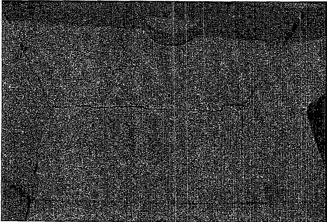
Settlement crack in ceiling of closet located under the stairs to the second level of the main house.
